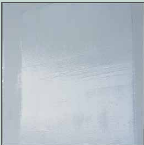
Surface finished with gloss paint (below)
