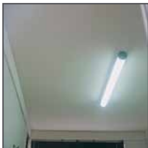
Ceiling fluorescent lights
